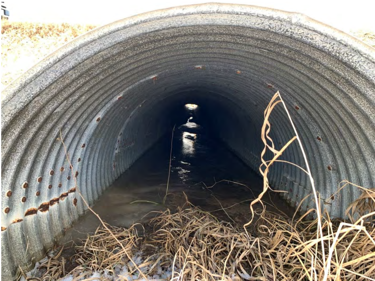
(S5) Structure 934386 - Culvert 934386XC – Culvert Barrell Deformation at Inlet
